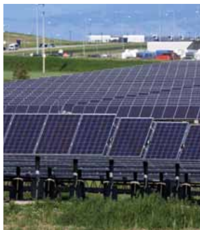
Solar PV panels
