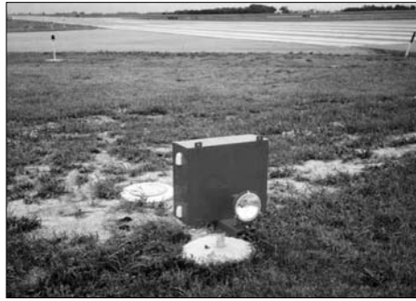
Runway end identifier lights (REILs)
